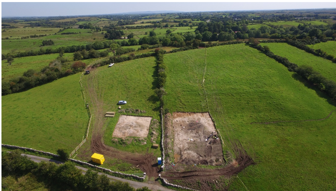
Fencing & Archaeological Excavations at Claggernagh East on the N5 Westport to Turlough Road Project
