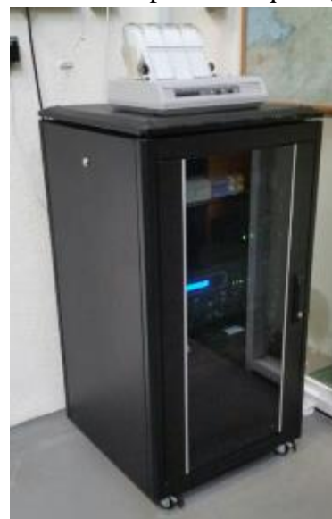
New Communication Equipment
