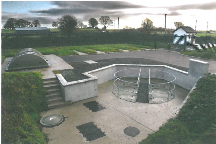
Mayo Abbey Sewerage Treatment Plant
