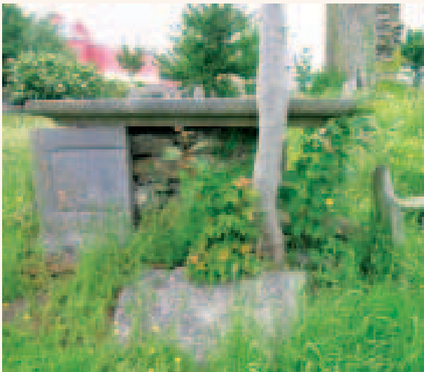
The damage caused by a Sycamore tree can be clearly seen in this graveyard
