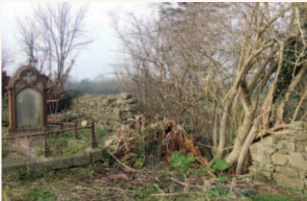
The planting of trees near graveyard walls should be avoided as their root system will eventually cause collapse, as shown here at Antrim, Co. Laois. There is a need to monitor self seeding trees in a graveyard and remove saplings near walls to avoid future long term damage and costs
