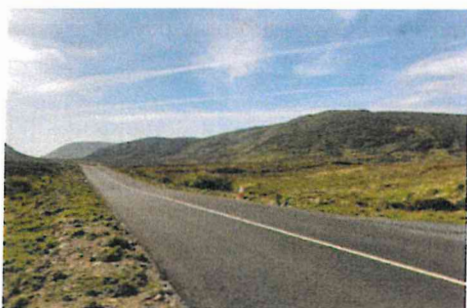
Regional Rd at Sligo Border, base course and temporary line marking completed in advance of HRA surface.
