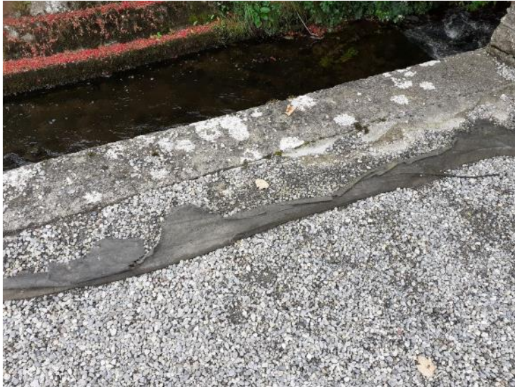
Plate 82: Some weed fabric has become exposed in the gravel area
